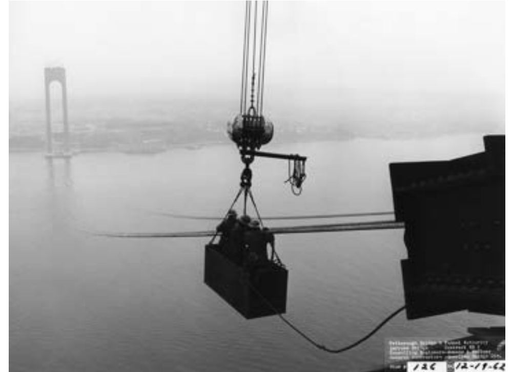
Figura 124. Construcción del puente de Verrazano-Narrows (foto Metropolitan Transportation Authority of the State of New York 1962, Wikimedia Commons)
